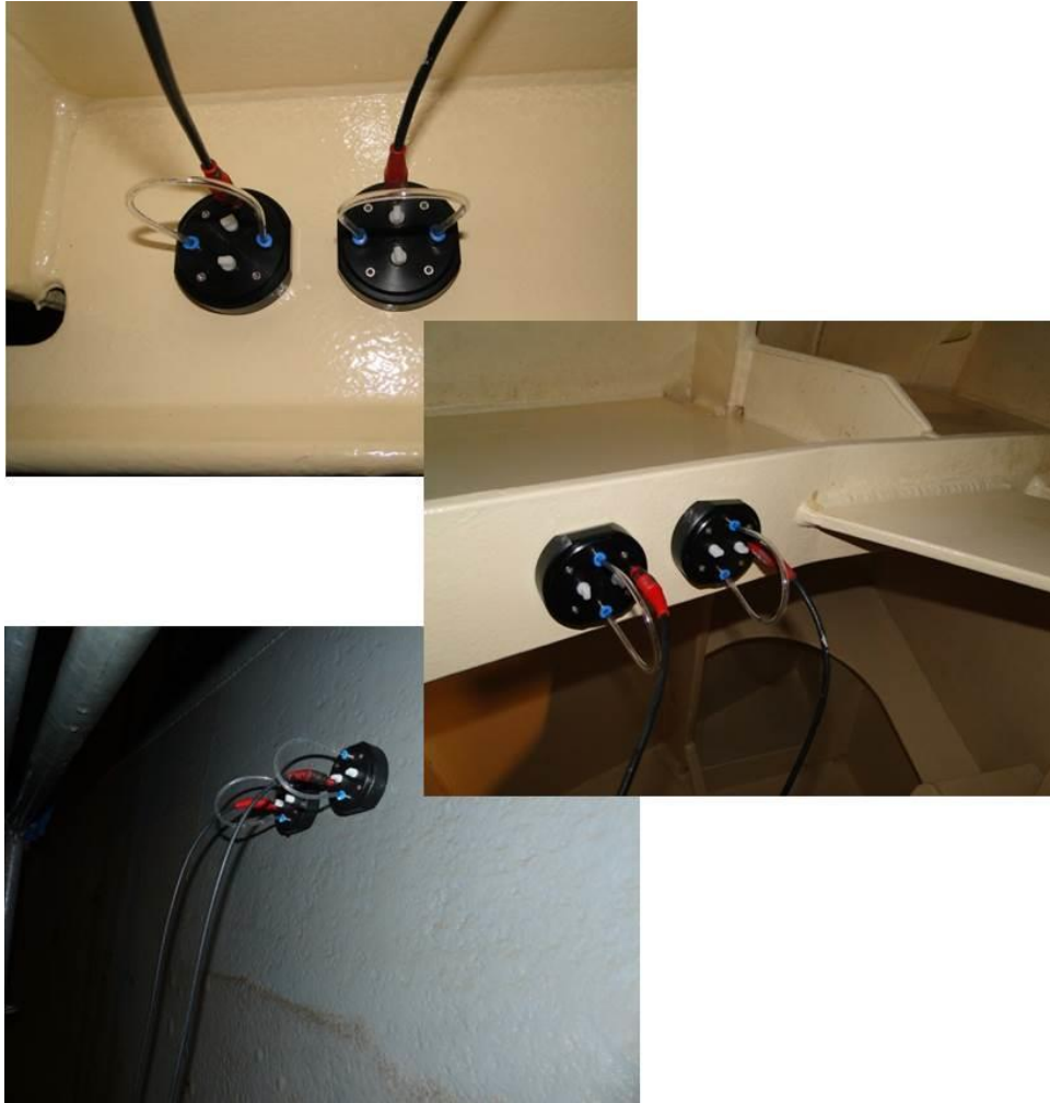
Figure 19: MCF Cells used during measurements in a ballas tank, bulk head, drinking water tank. [Photo's courtesy of ENDURES]
